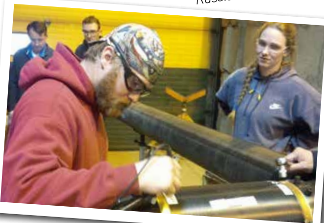
USA - Sleeve Manşon Kaynak Uygulaması USA - Winconsin Nuclear Power Plant Sleeve Coupler Installation
